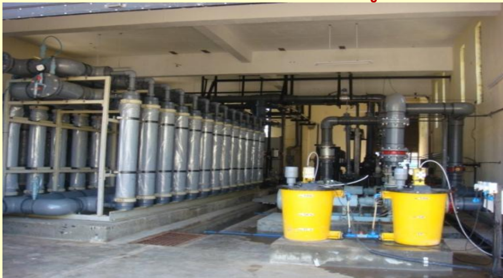
5280 Cubic meters/day ultrafiltration membrane based plant in BARC Facility (Source: Article 1; page 2)
