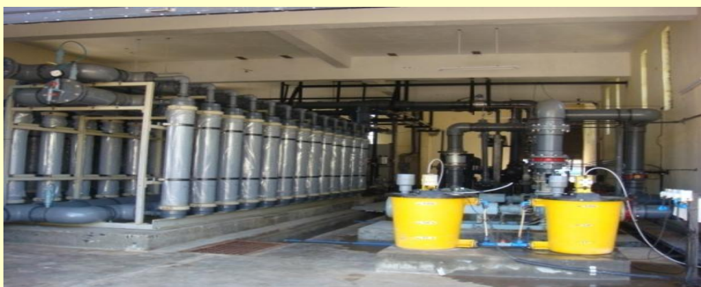
Fig.1: 5280 Cubic meters/day Ultrafiltration membrane based plant in BARC Facility
